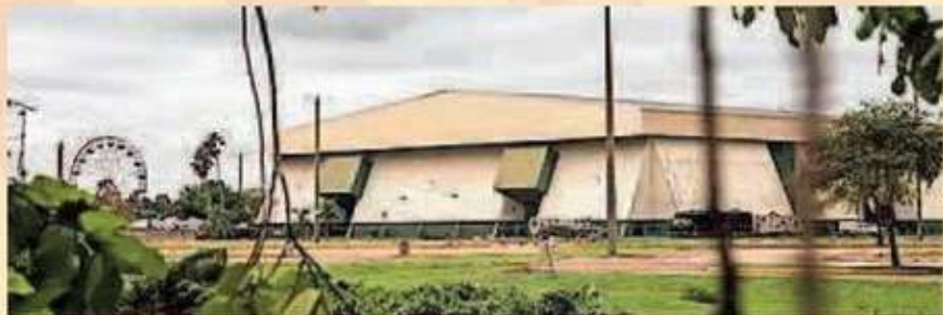
The Lee Civic Center is in rough shape, with bleachers that can't be used and other problems. Lee County is evaluating its future. ANDREW WEST/THE NEWS PRESS
