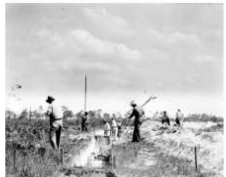
Construction by the FERA of north River Road between Alva and Olga - Lee County, Florida 1935
